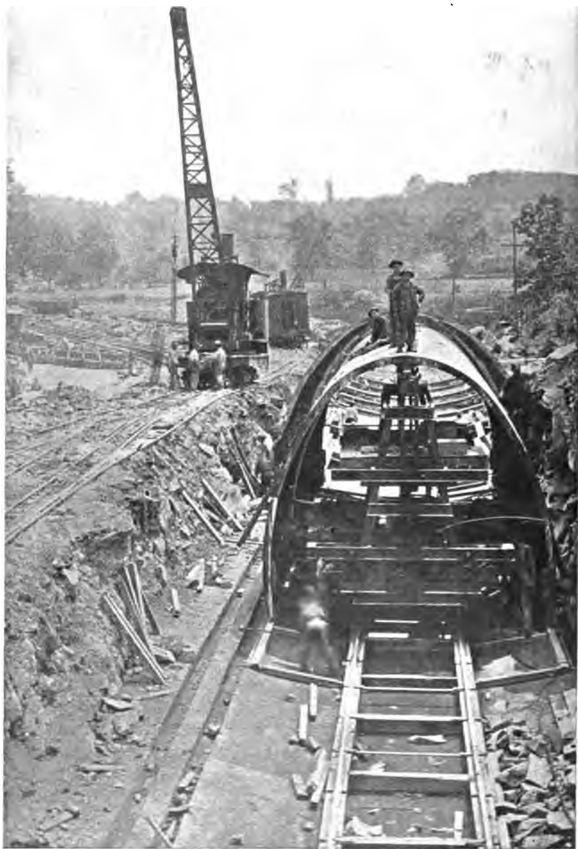
PLATE 69. —Contract 11. Construction of Cut-and-cover Aqueduct on Section 1. Shows Steel Form and Carriage; also Locomotive Crane Used to Place Concrete, Move Outside Forms, and Assist in Excavation.
